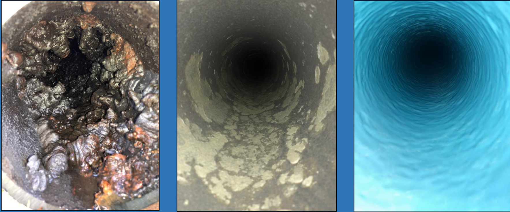
Left, Iberville St. pipe before cleaning, center, after cleaning and right, after lining with BluKote.
